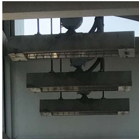
Platform Light & Heaters (A Line Shown)
