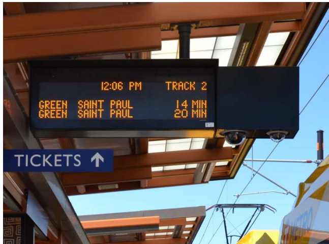
Variable Message Sign (VMS) (METRO Green Line Shown)
