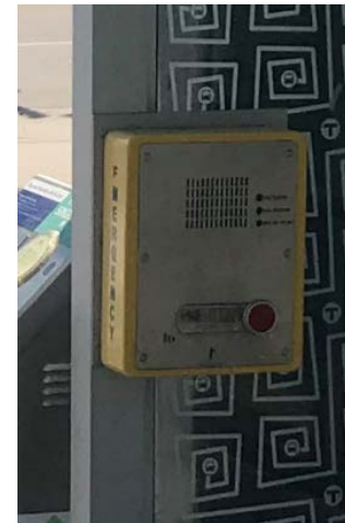
Emergency Telephone (A Line Shown)
